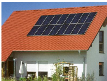
Fig. 4: Roof-mounted solar cells.
