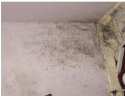
Fig. 2: Mould formation on walls and ceiling as result of poor thermal insulation and ventilation.
